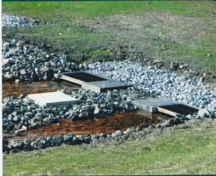
Passive AMD treatment system
