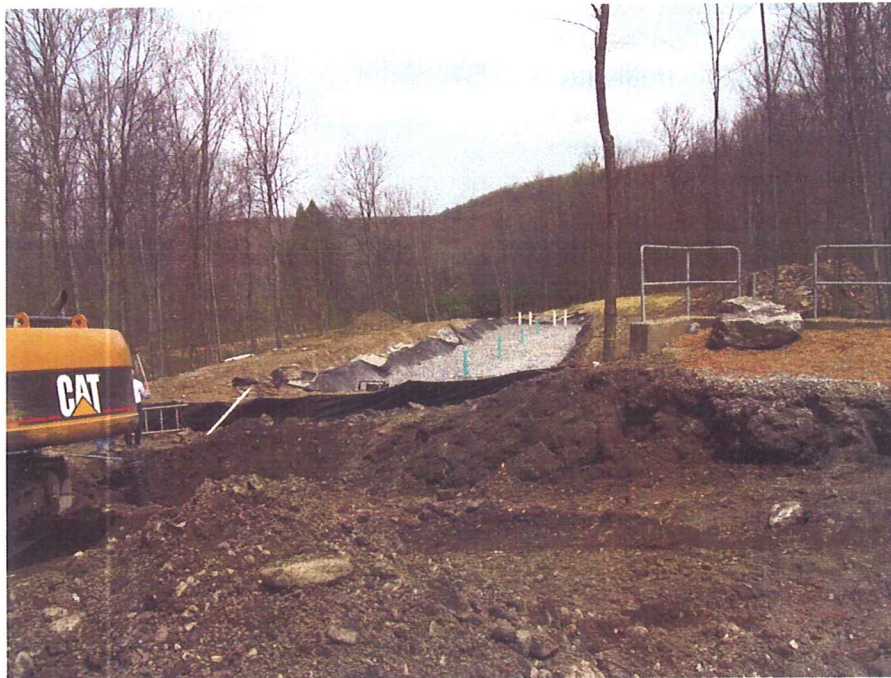
Limestone and Monitoring Ports – May 2006
