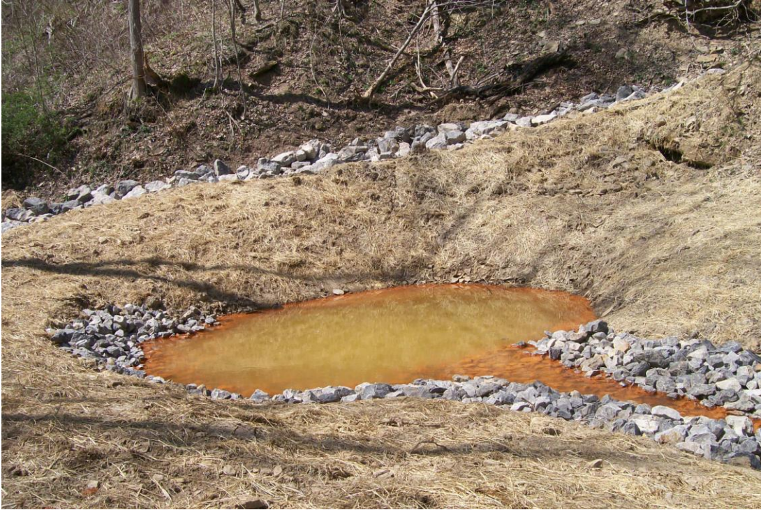
Picture 7: Completed impoundment of mine discharge and beginning of delivery channel, also showing surface water diversion channel
