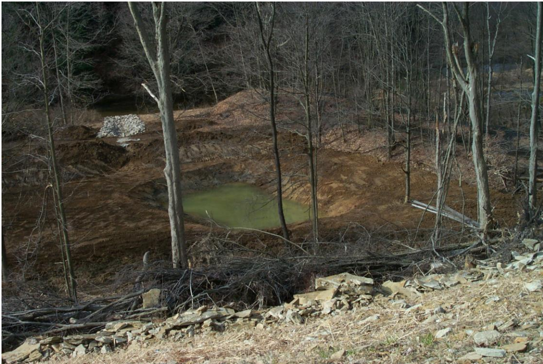
Picture 6: View of third cell showing excavated area and outflow with 24-inch CPP
