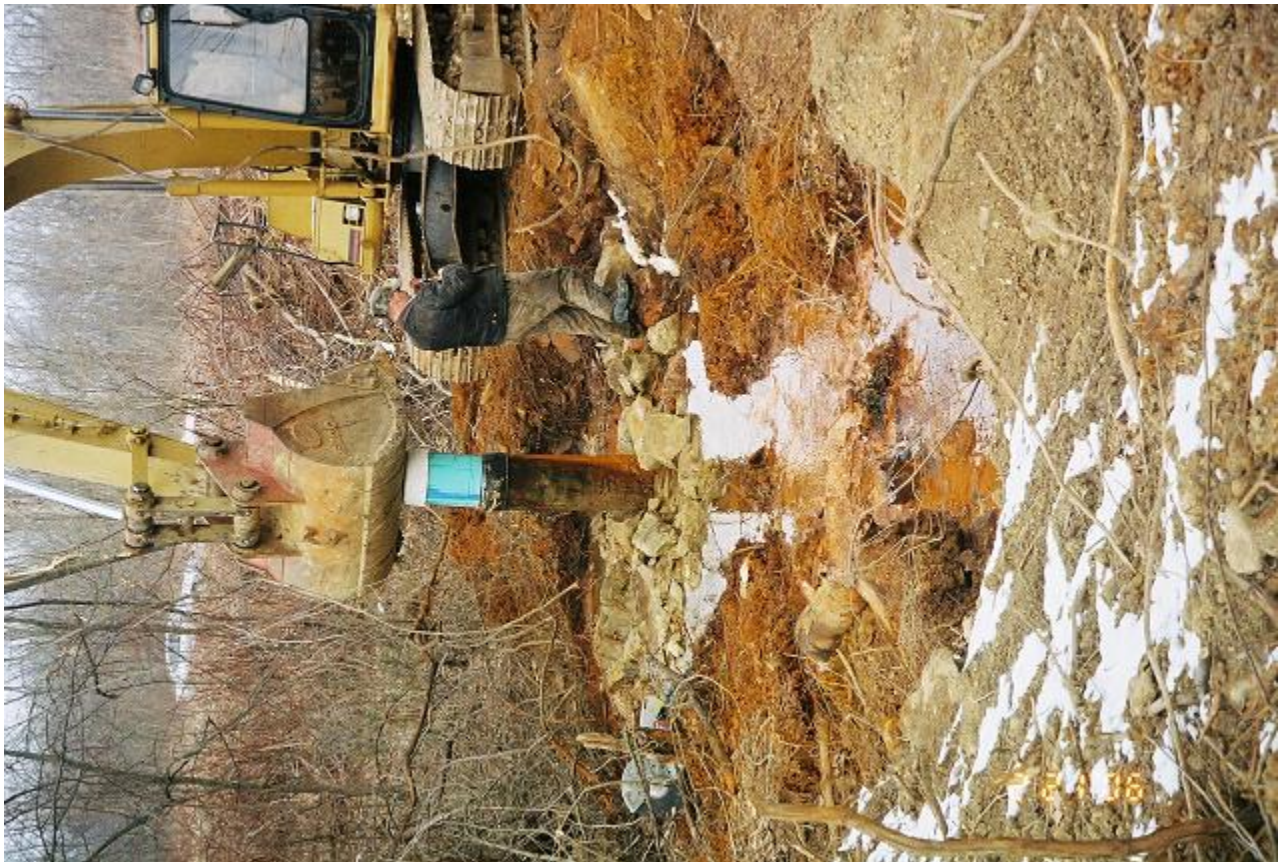
Rotated view of Main Discharging Borehole Pipe with "Bubbler" in foreground
