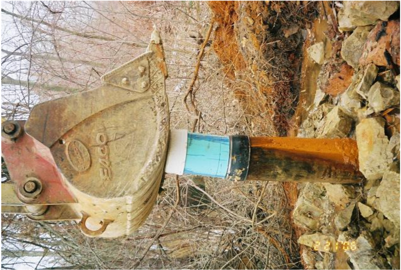
Rotated view of Main Discharging Borehole Pipe with Fernco, Pipe Stub and Cap in Place
