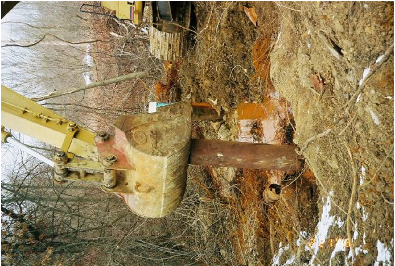
Rotated view of “Bubbler” with Casing Pipe being driven in to seal the outflow
