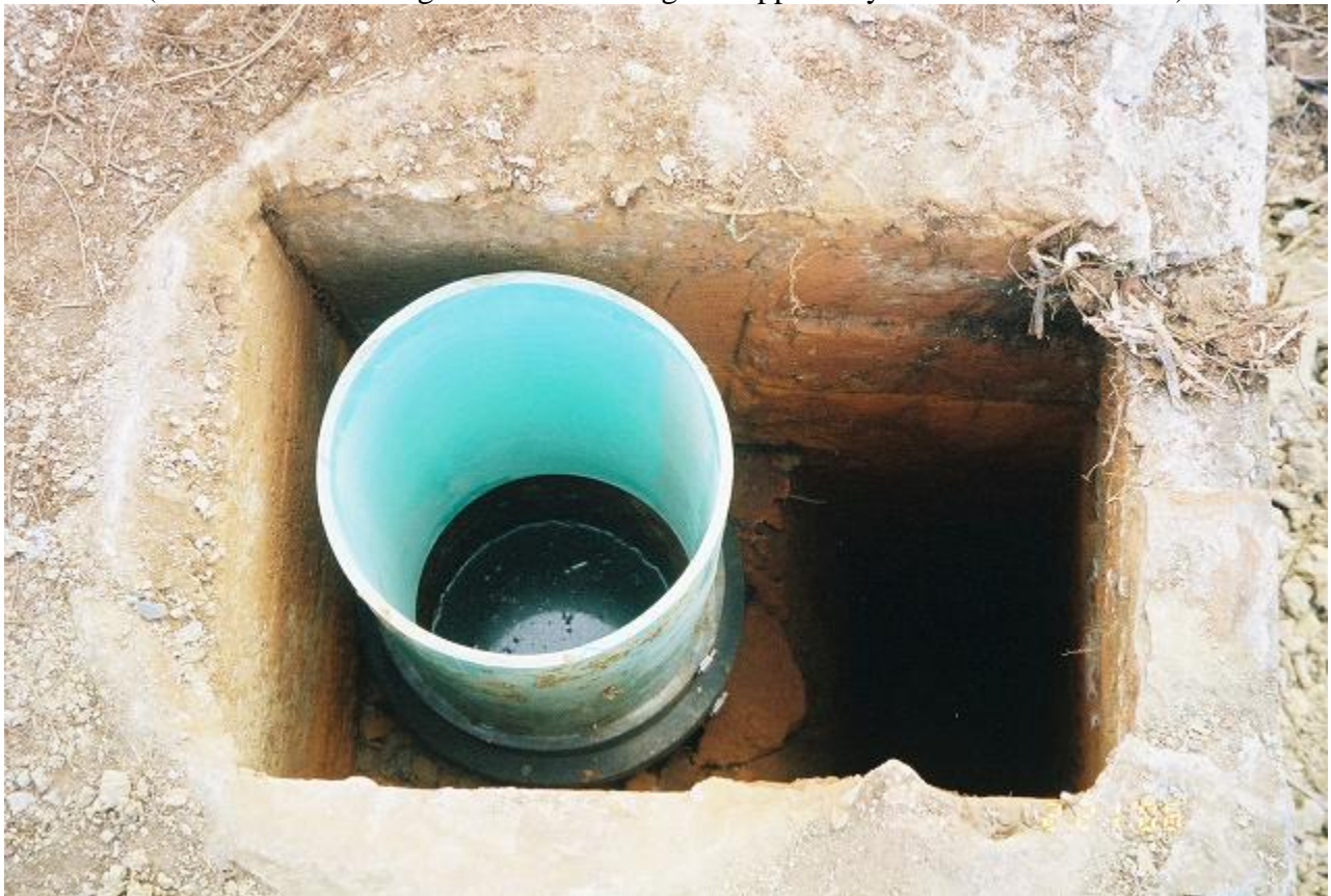
View inside the “Manhole” structure with a Fernco fitting and PVC pipe stub
