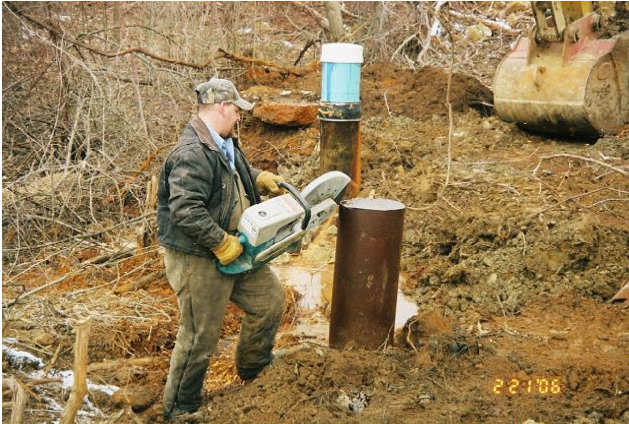
Grinding the top of the casing pipe prior to sealing the “Bubbler” discharge pipe
