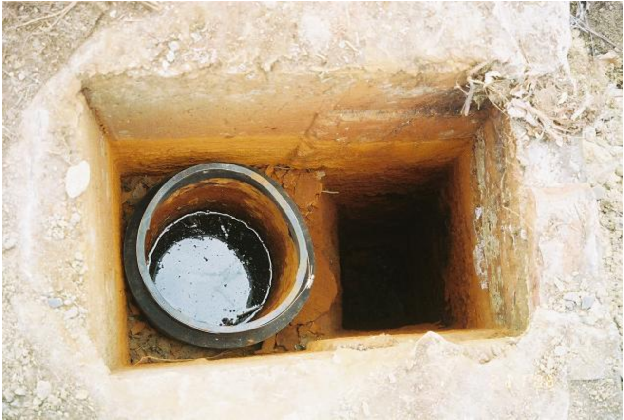
View inside the “Manhole” structure with a Fernco fitting over the pipeline on the left side (Note that the rectangular area to the right is apparently an overflow structure)
