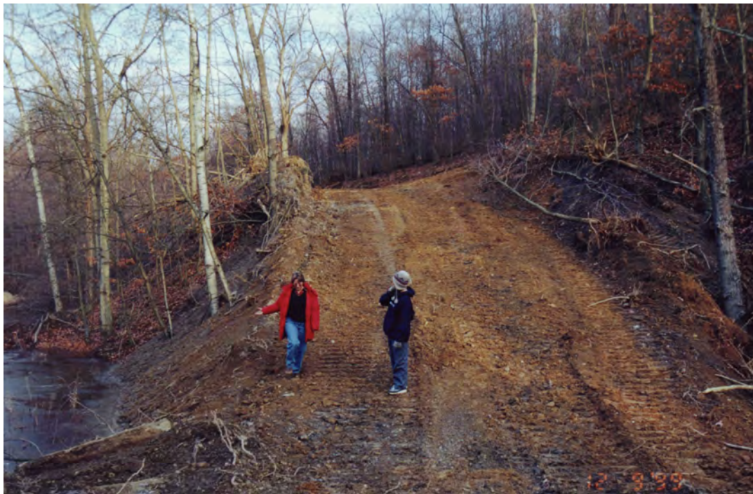
Abandoned Brookville pit and existing highwall. Coal refuse from the Goff Station Restoration Area is incorporated with alkaline, circulating, fluidized-bed coal ash from Scrubgrass Generating Plant (Kennerdell, PA) and placed into pit. (Pictured: M. Dunn, D. Peart)
