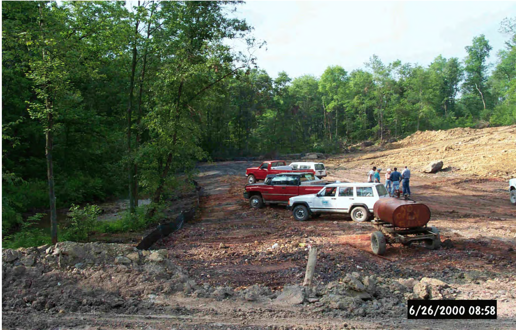
Project area after coal refuse has been removed. Future site of forested and emergent wetland.
