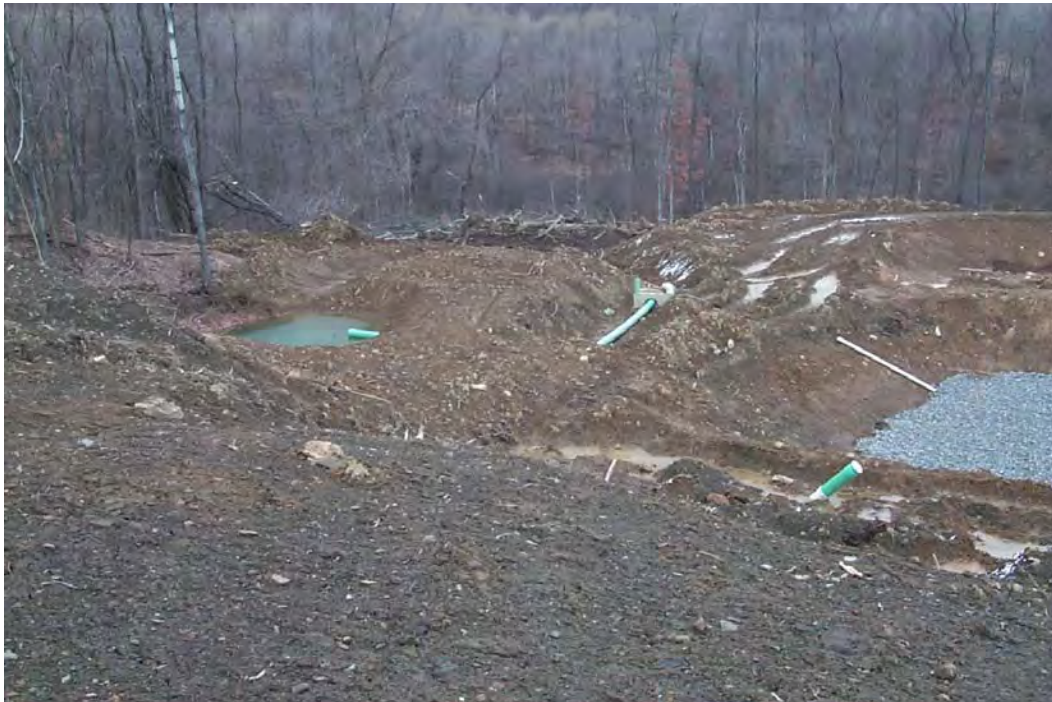
View of a portion of the ST 40/40A/42 collection system. Note ST42 pool far left, splitter box center, and clean out far right.
