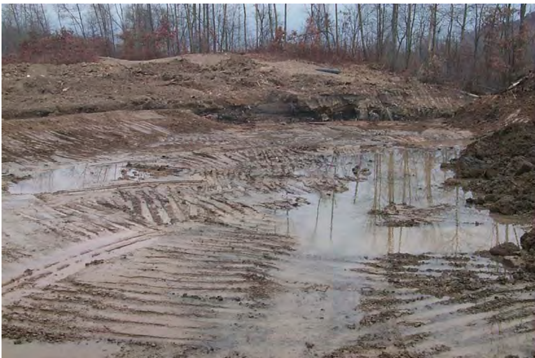
Section of ST41 Upper Wetland excavated to appropriate depth for the placement of hydric substrate. Berm of collection ditch visible to the left. (11/8/00)
