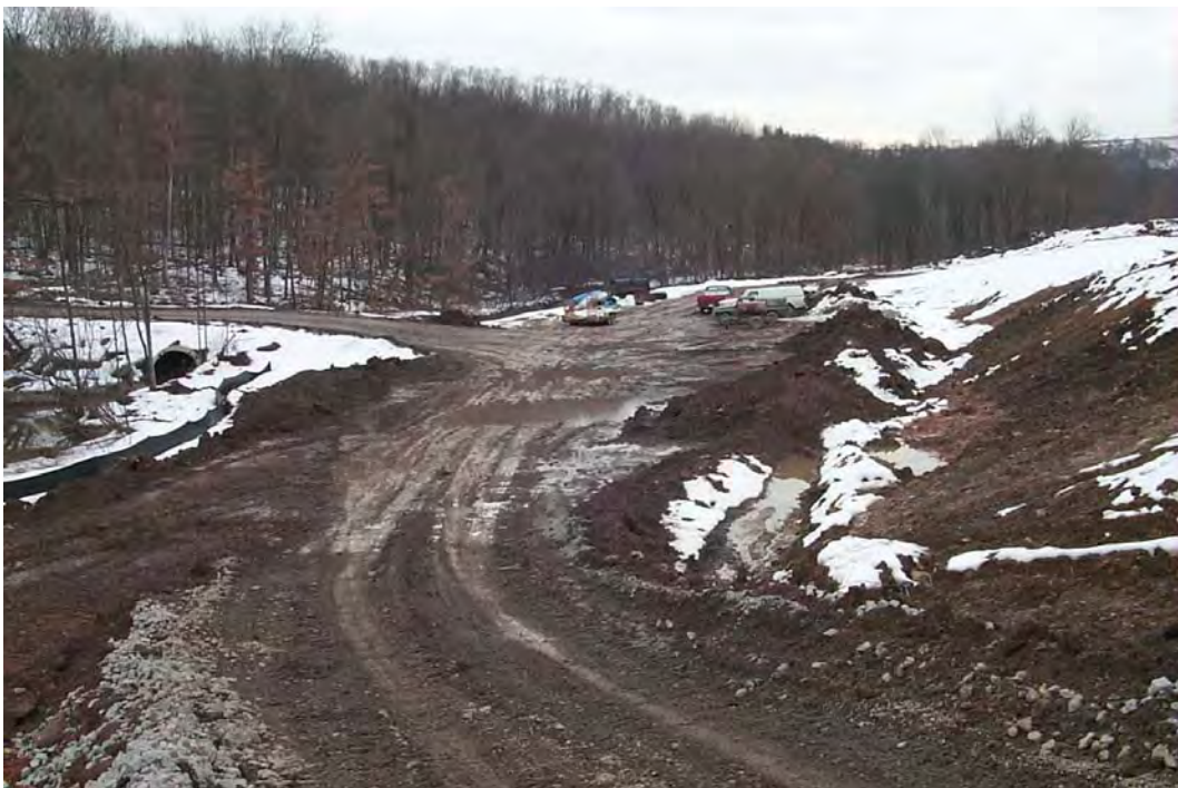
Basin for footprint of the finishing wetland, final component of the passive treatment system. (2/8/01)
