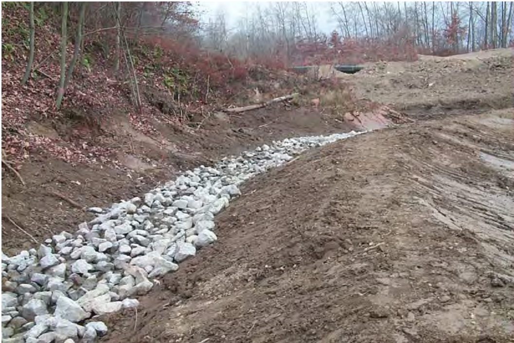
Collection ditch for seeps from abandoned underground mine workings to be treated by the ST41 Upper Wetland. (11/8/00)
