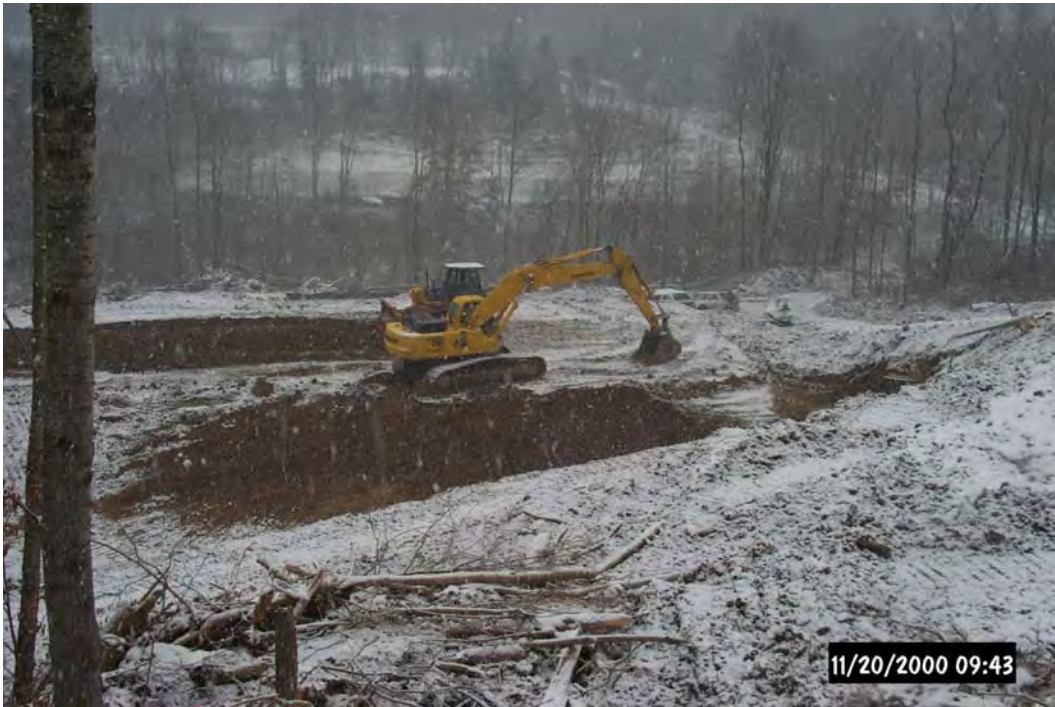
Construction of Vertical Flow Ponds #3 & #4 for ST40/40A/42 with the option of including ST41 by Quality Aggregates.
