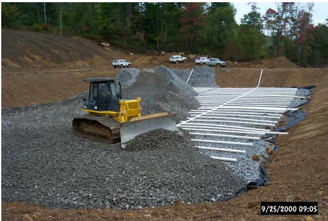
Placement of 3000 tons of AASHTO #1 limestone in Vertical Flow Pond #2 for ST38/39. Note the flushing system with additional clean outs (first known of this design in Pennsylvania).
