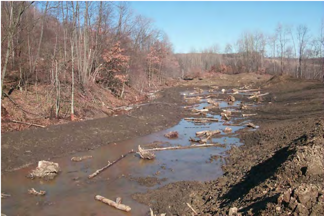
ST41 Upper Wetland following placement of hydric substrate and woody debris. Standing water is from the spring thaw. Flows from ST41 are not yet entering the treatment wetland. (3/22/01)
