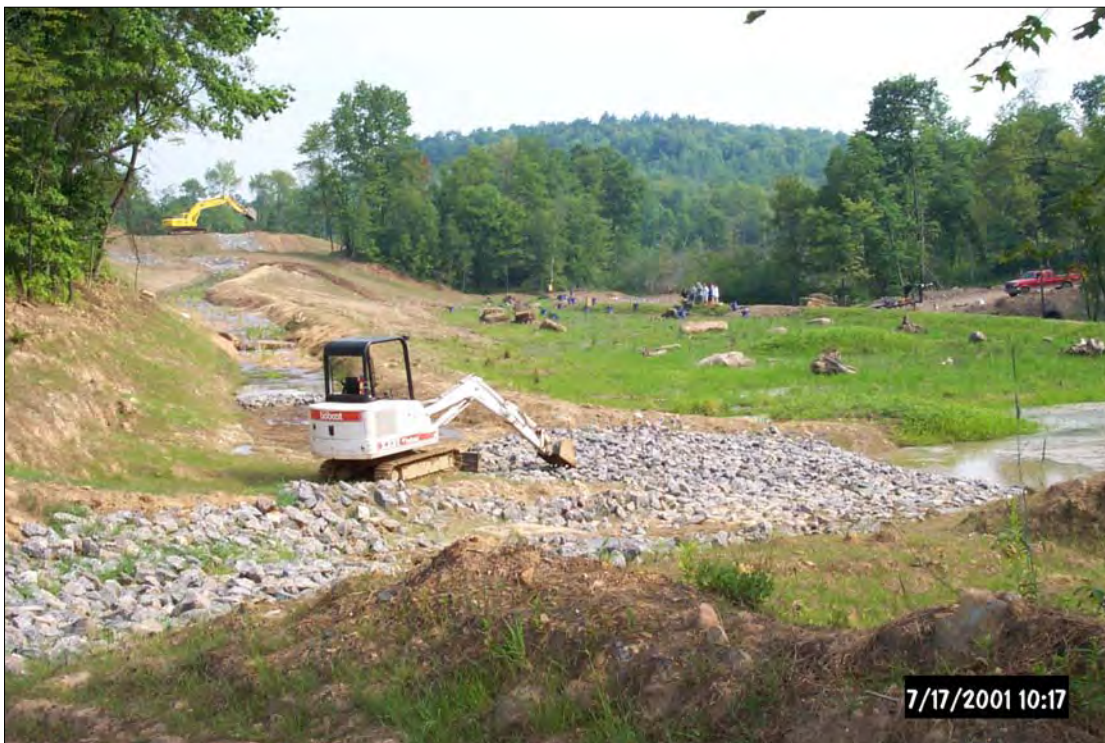
View looking towards the final wetland (Center Right) and the Bioswale (Center Left) during planting of the final wetland.
