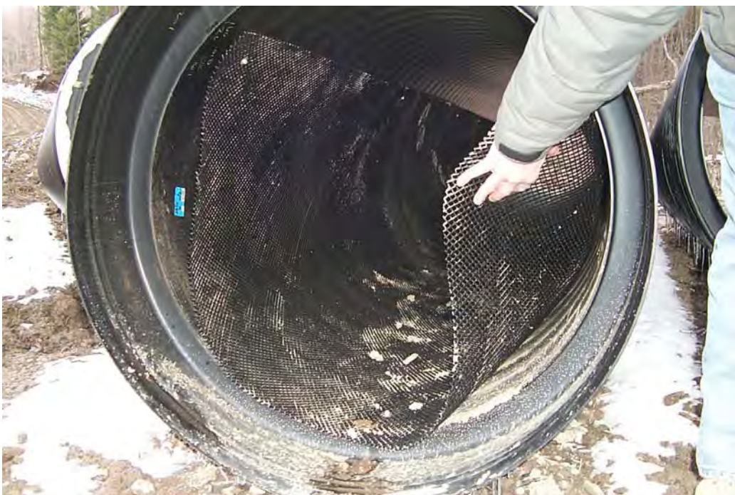
Tex-net (plastic netting) was used to line inside of the tunnel and HDPE manhole to provide foot-holds for bats. (3/28/01)
