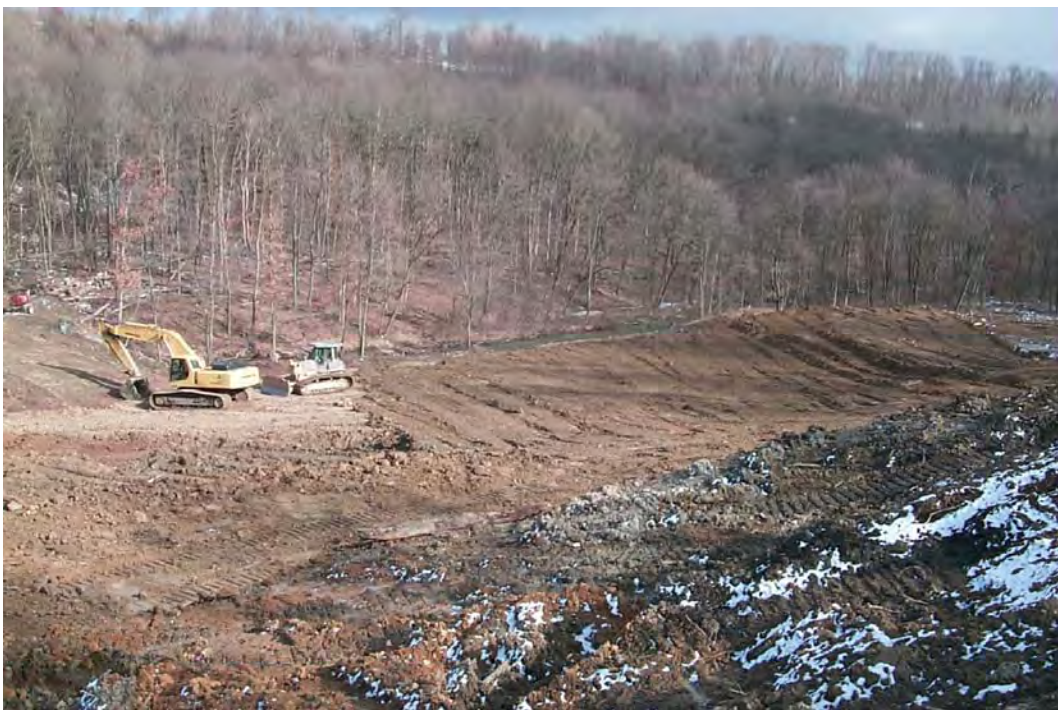
Placement of clay to seal the floor of the final polishing wetland. Murring Run can be seen in center of the photo. (3/28/00)
