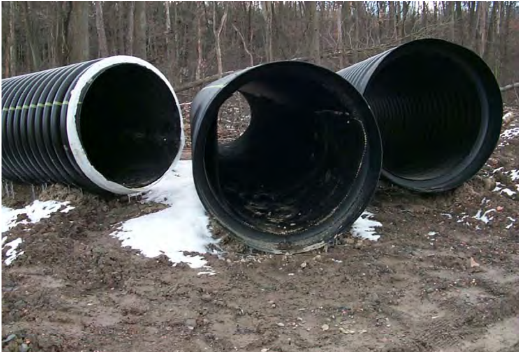
Culvert pipe was used to provide a 60-foot tunnel entry into the bat hibernaculum. (3/28/01)
