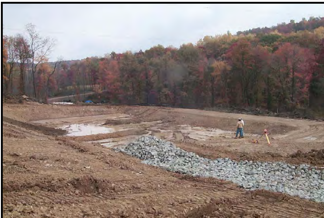
ST 38/39 wetland basin with flow diversion structures and limestone spillway inlet. Laser level was used to monitor elevations of the wetland basin during construction. (10/16/00)
