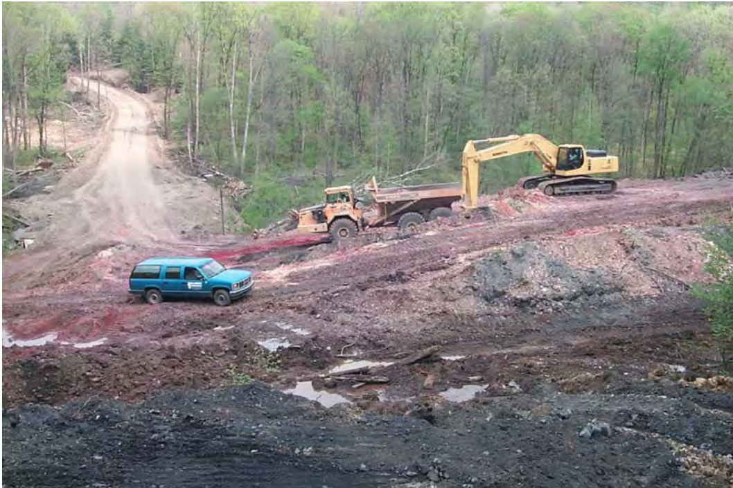
Gob removal in progress. The footprint of the removed gob pile is the location of the finishing wetland. (5/12/00)
