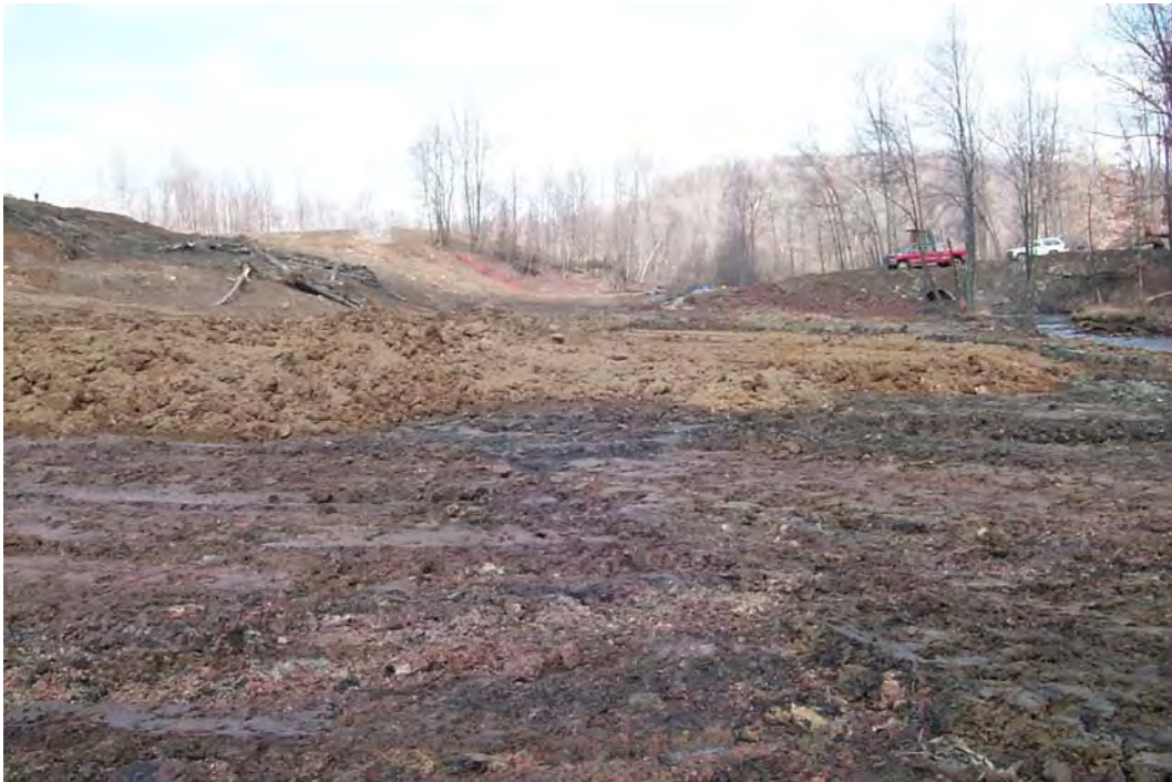
Placement of clay over remaining coal refuse to seal the floor of the final wetland. (3/23/01)
