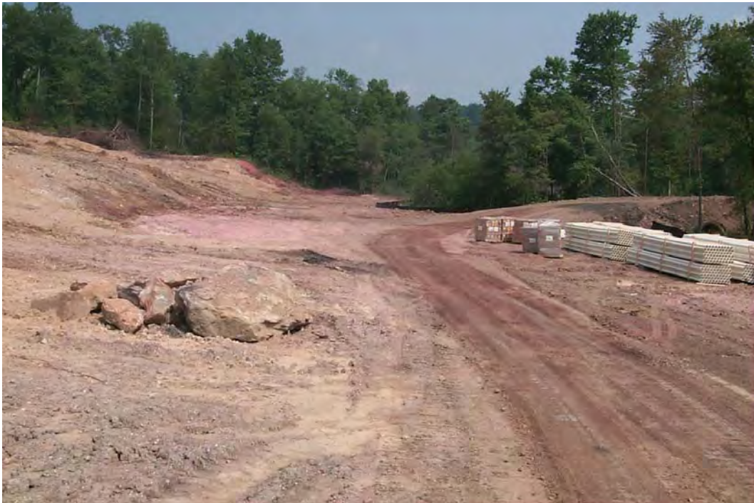
Basin for footprint of the finishing wetland, final component for ST38/39, ST 40/42. And ST 41 discharges. (7/28/00)
