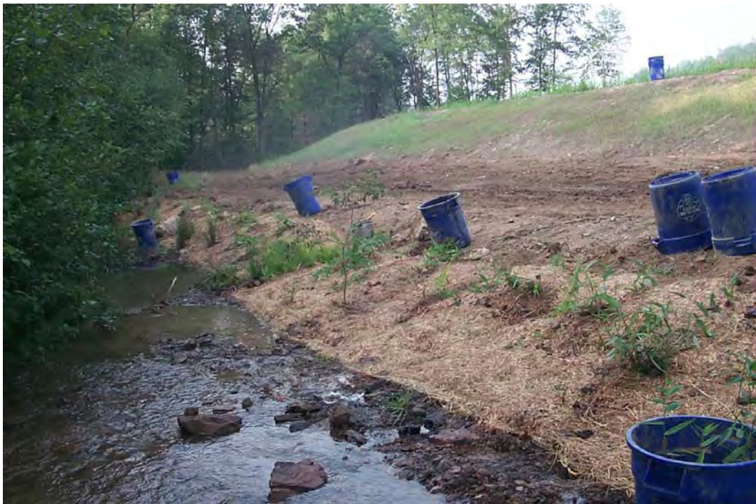
Planting of riparian area (south of stream crossing) following addition of soil, seeding, and installation of willow wattles and erosion control fabric. (8/9/01)
