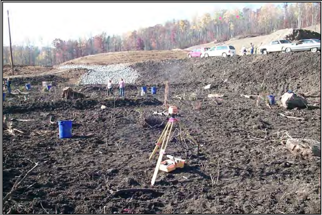
ST 38/39 wetland planting. Laser level was used to transplant vegetation to appropriate elevations. (10/21/00)
