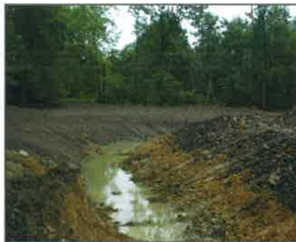
A trapezoid channel with an eight foot depth, 25 foot top width and a length of 150' served as the settling basin for precipitated metals
