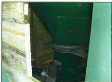
The base of the silo was enclosed to protect the doser from rain. Rain water contacting the hydrated lime causes the lime to cake, rendering the dosing system inoperable.
