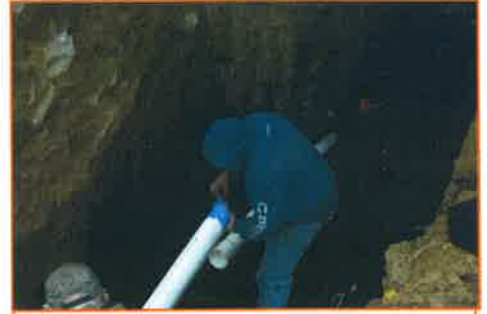
Four inch schedule 40 pipe was inserted into the bore and grouted with concrete.
