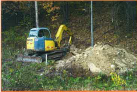
We had to excavate eight feet to expose the coal out crop.
