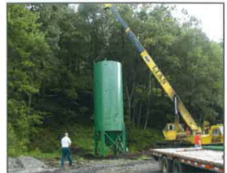
A fifty-ton crane was used to place the silo. Adequate room is needed for silo delivery and placement.
