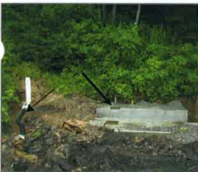
One foot square metal plates were anchored into the concrete. The silo legs will be welded to these plates to secure the unit. Mine flow is diverted around the worksite.
