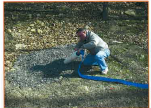
After backfilling . The sealed pipe easily accommodates the discharge from our three inch trash pump.
