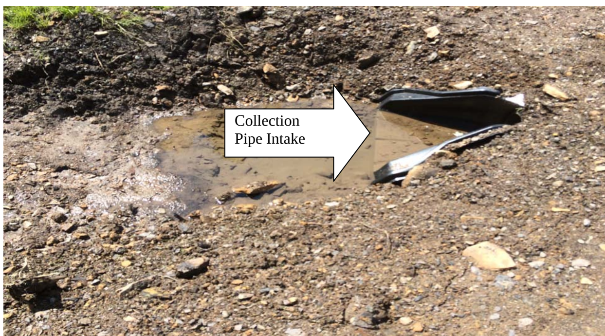
Photo 9: Collection Pipe Intake (Prior to Seeding)
