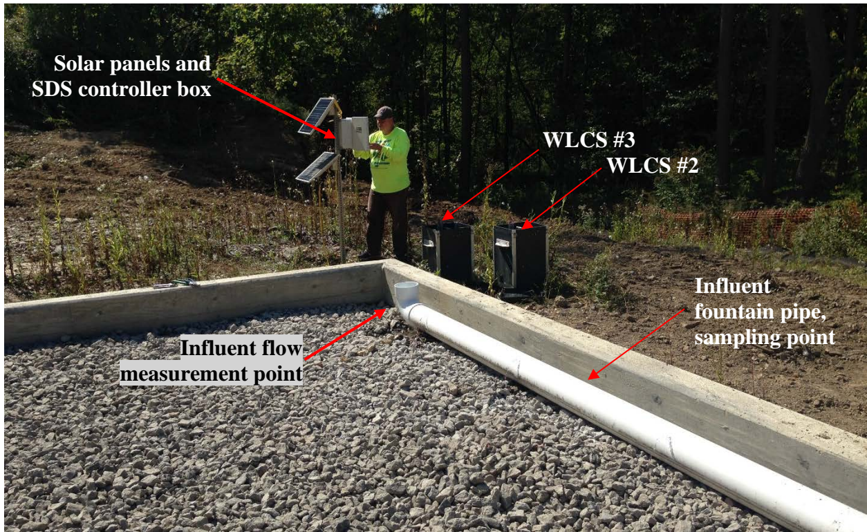
Photo 5. Influent fountain pipe and water level control structures
