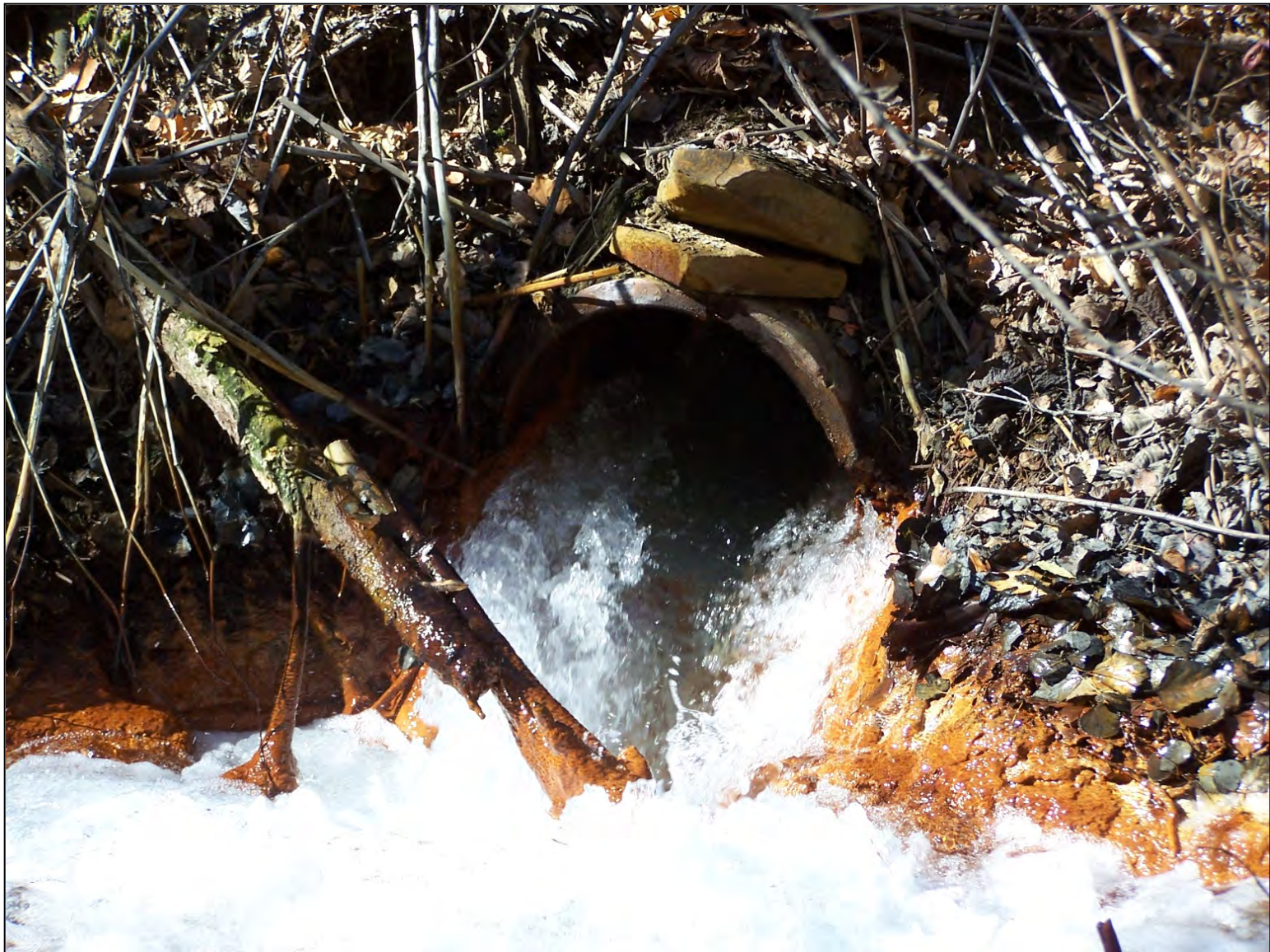
36" Diameter pipe near the top of the abandoned Maryland No. 1 Mine shaft collar discharging Acid Mine Drainage (AMD) since December 1963.
