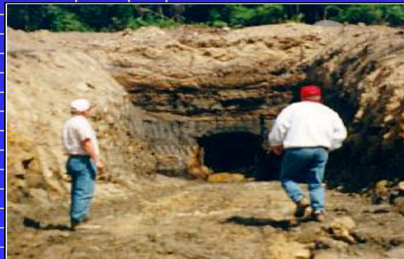
One of the three mine openings that was sealed; the acid mine drainage that is collected from the openings will be treated in phase 2.
