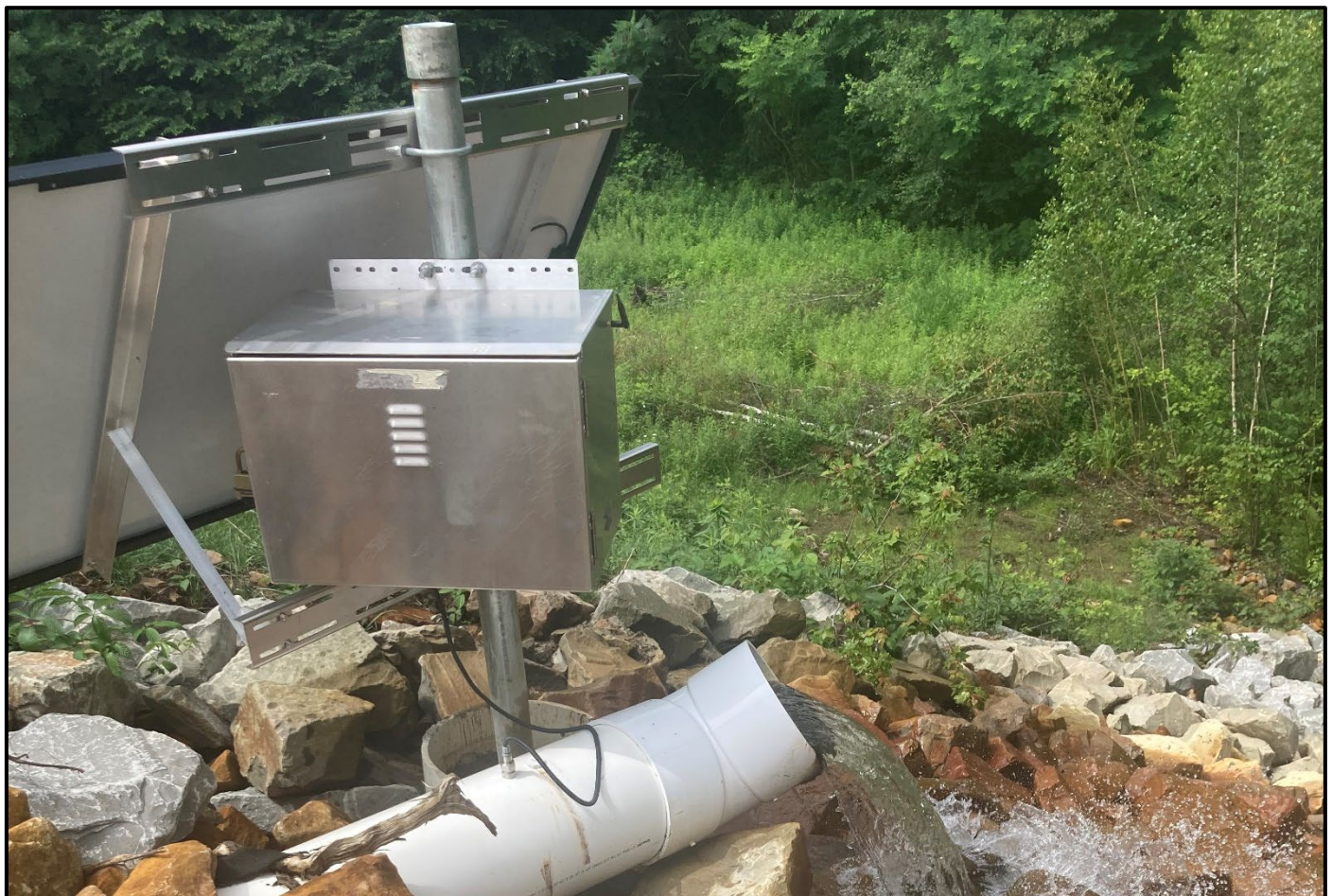
Top: JFVP1 and JVFP2 riser pipes discharging to SP3 with baffle curtains. (9/8/22)
