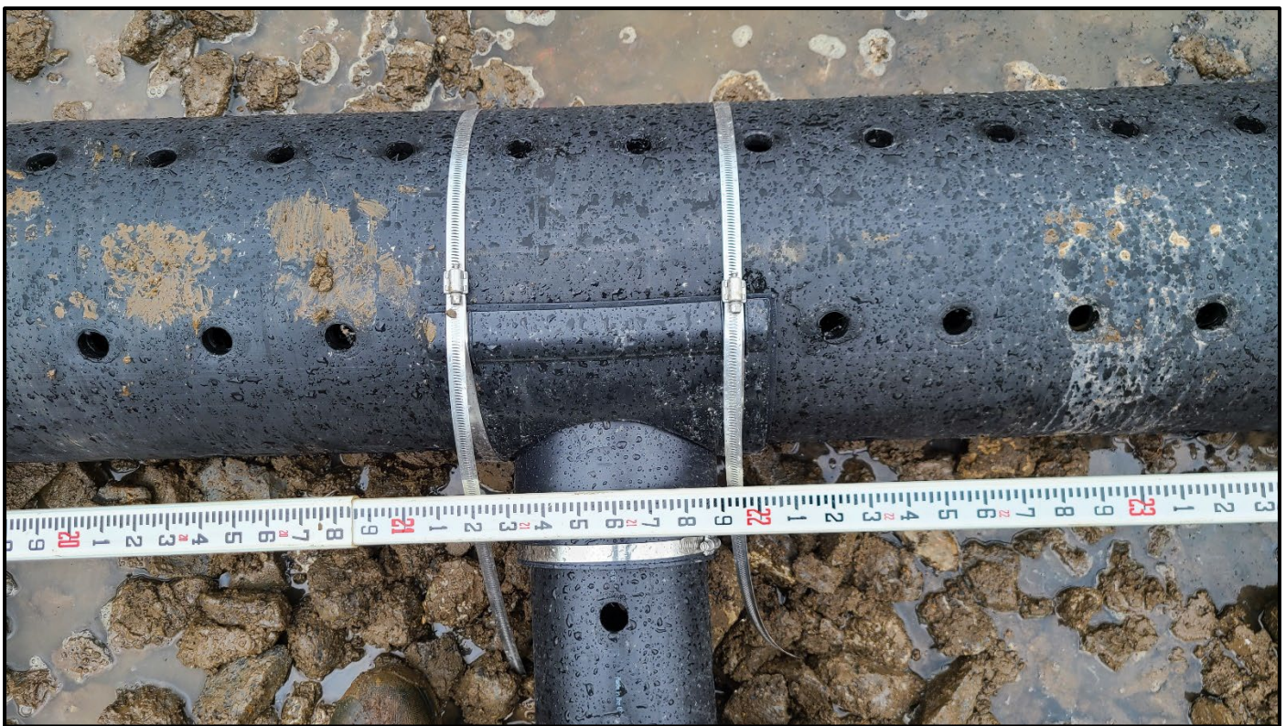
Top: 12-inch DR-26 HDPE header pipe with 12-inch HDPE tee connected with 12-inch non-shear flexible couplers with 6-inch DR-17 perforated lateral. (4/29/21)
