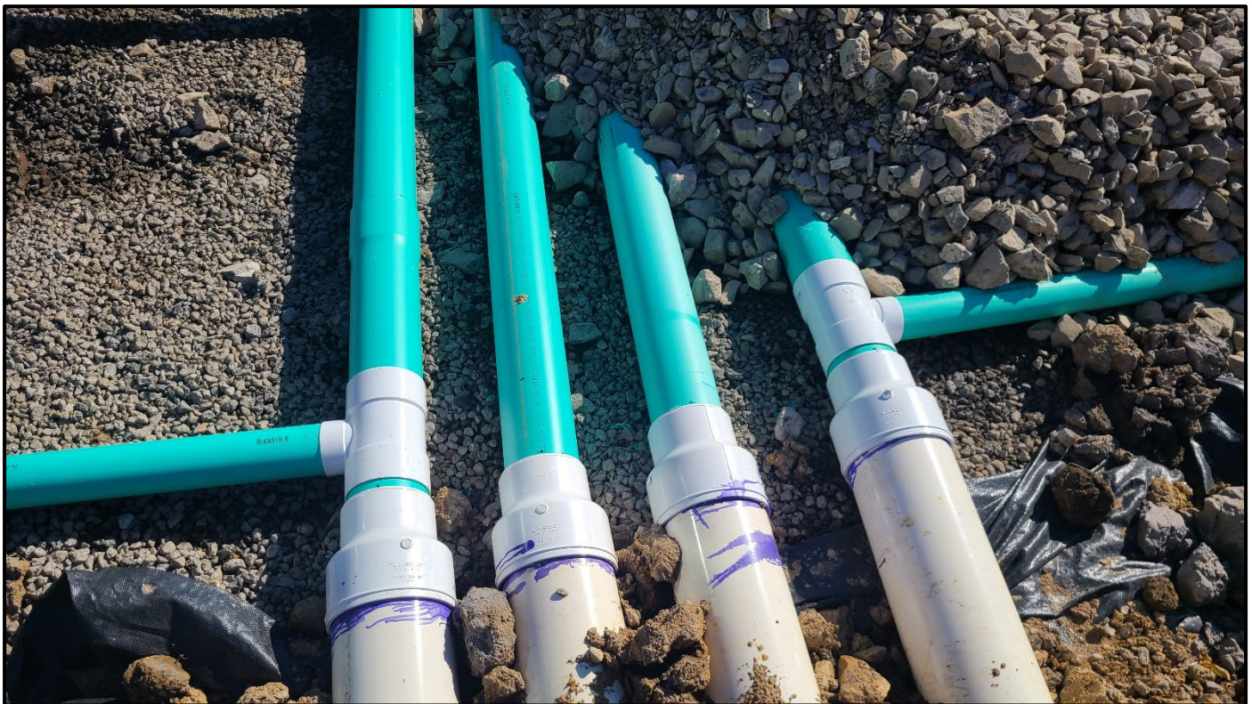
Top: Jennings-type Vertical Flow Pond underdrain with solid 6-inch SDR35 PVC header pipes and perforated 4-inch SDR35 PVC lateral pipes. To the right is the mix of 2,800 tons of limestone, 700 CY of spent mushroom, and 1,400 CY of wood chips. (10/20/21)
