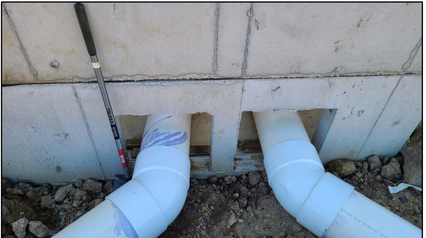
Top: Three-Way Flow Splitter with Agri Drain Smart Drainage System structures connected to 12-inch SCH40 pipe that flow into AFVFPs. (2/16/22)
