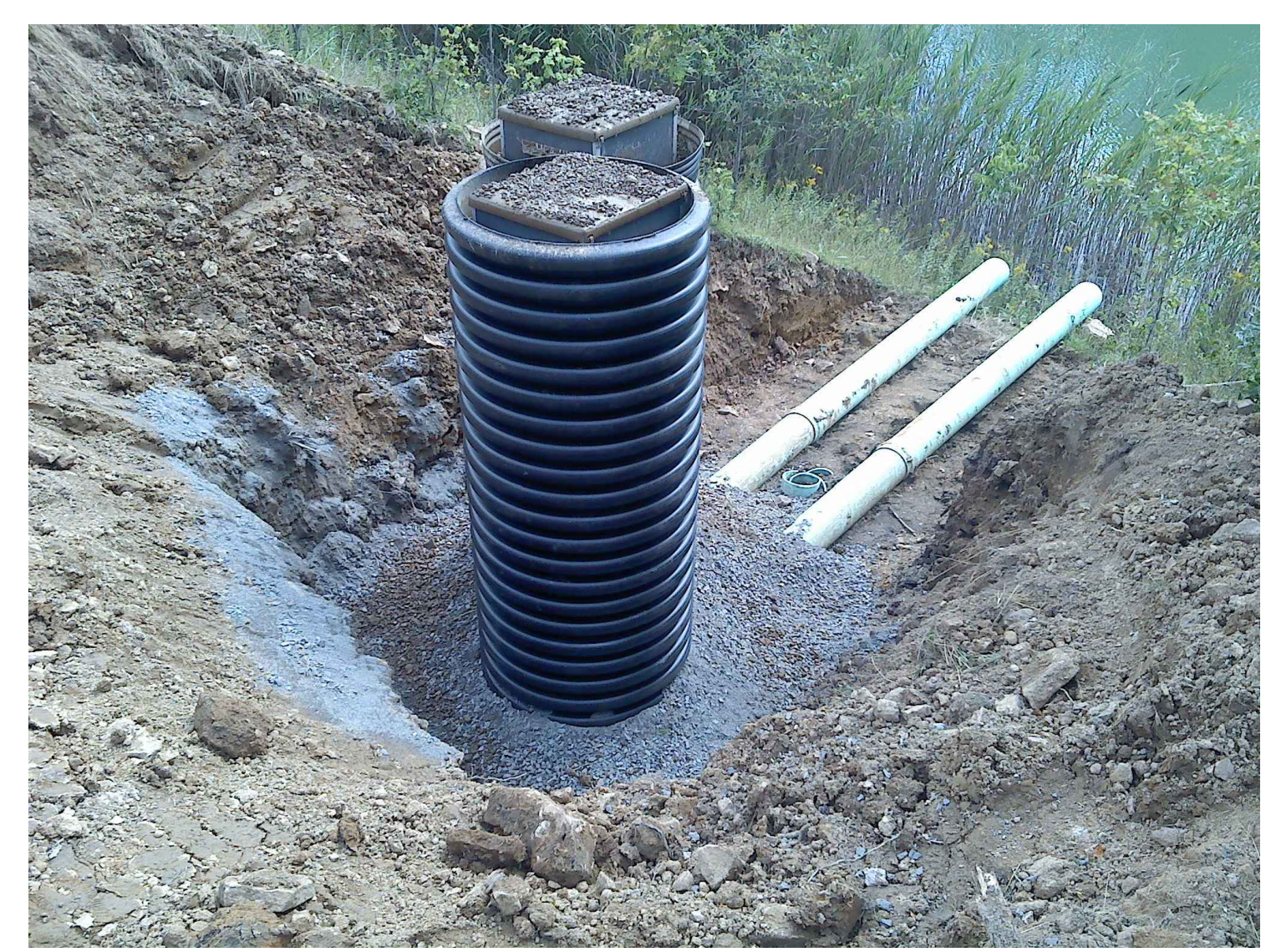
Note: The WLCs will have corrugated smooth wall pipe placed on outside of the boxes to prevent distortion of the WLCs during backfilling. The pipe should extend from top of pipe at bottom of the box to one foot above the surface. The annulus shall be filled with AASHTO #57 aggregate
