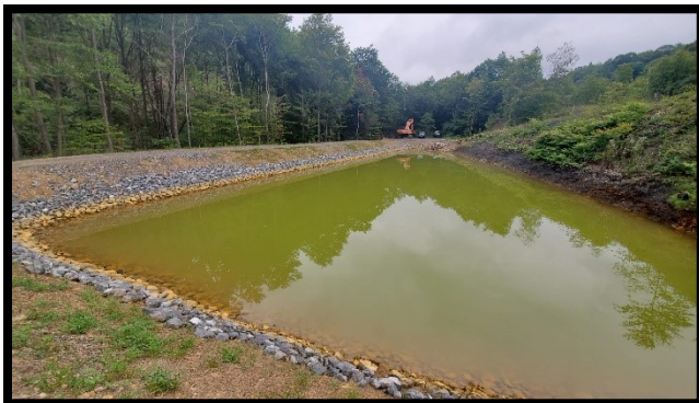
Top Left: Excavation of the HP and removal of existing limestone from FeAlMn Bed. (5/27/2020)
