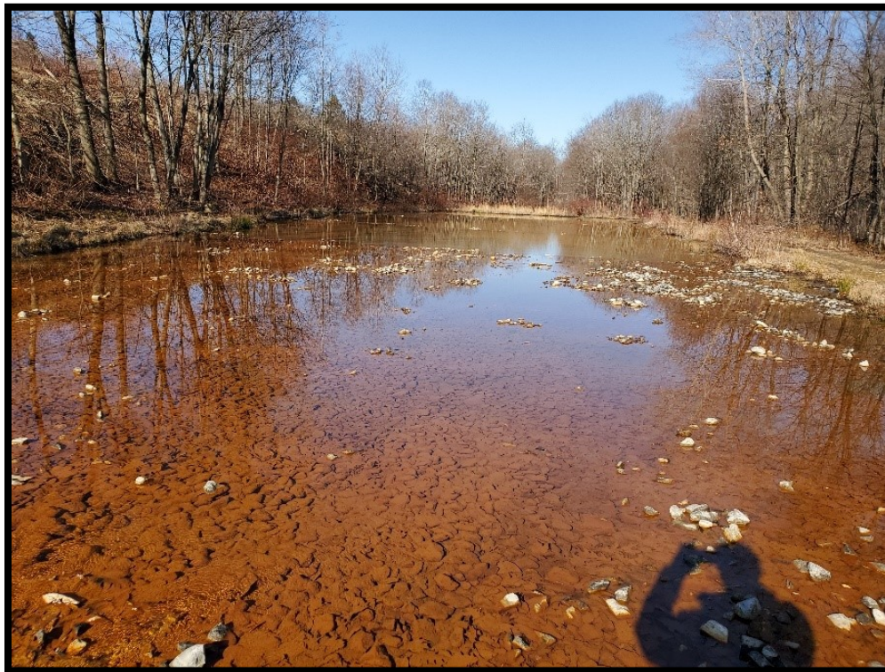
Top Left: Puritan discharge inlet to the original PTS, the system inflow was restricted to about 100 gpm. (3/5/2020)
