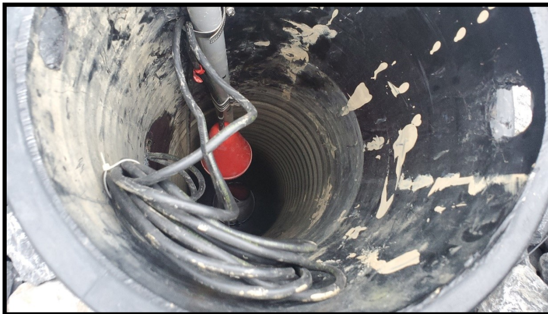
Top Left: A custom floating skimmer is used to dewater SP1 to help buffer flow rates through the system to allow for better treatment and more stable discharge rates into the Trout Run. (9/10/2020)
