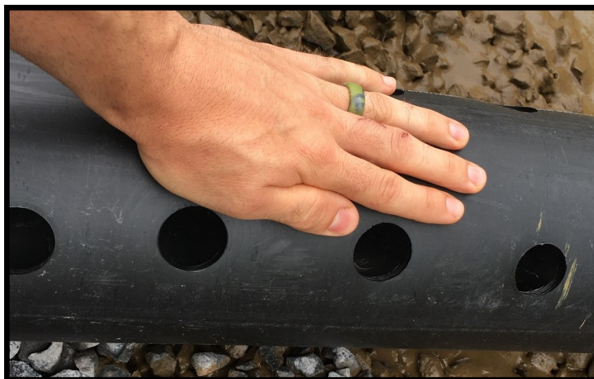
Top Left: 6" perforated HDPE underdrain in AFVFP1 prior to being filled with limestone. (5/27/2020)
